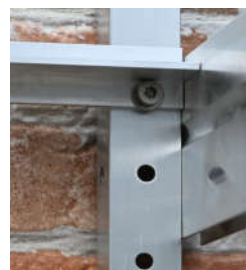
Bolt sits below staging rail
