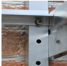
Bolt sits below staging rail
