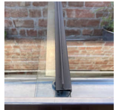
Roof glass overlapping
