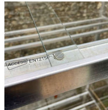
Roof glass overlapping
