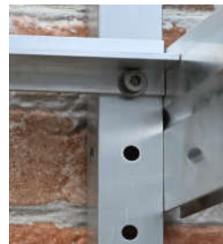
Bolt sits below staging rail
