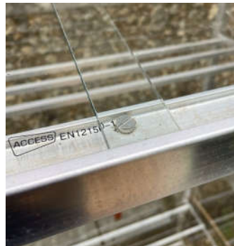
Roof glass overlapping
