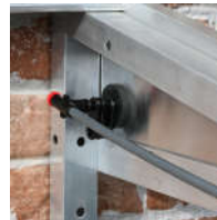
Inlet and link pipe
