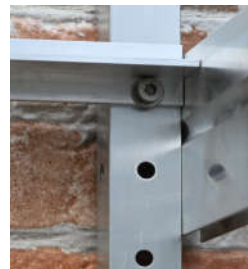
Bolt sits below staging rail
