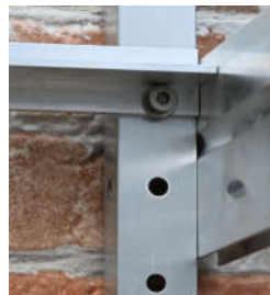
Bolt sits below staging rail
