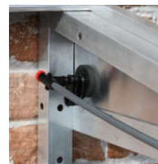
Inlet and link pipe
