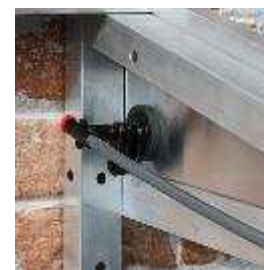
Inlet and link pipe
