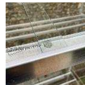
Roof glass overlapping
