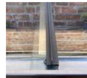
Roof glass overlapping
