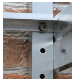
Bolt sits below staging rail
