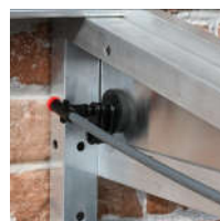
Inlet and link pipe
