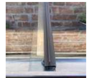
Roof glass overlapping
