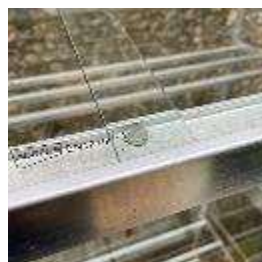
Roof glass overlapping
